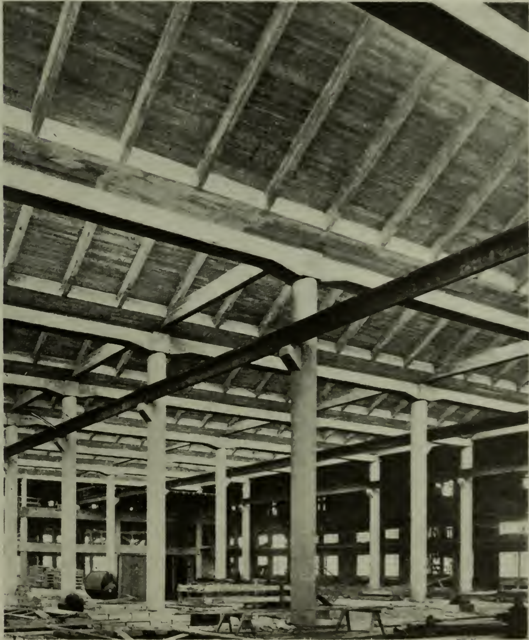
REINFORCED CONCRETE BOTTLING BUILDING, ST. LOUIS - TOP STORY, SHOWING SAW TOOTH ROOF CONSTRUCTION.
